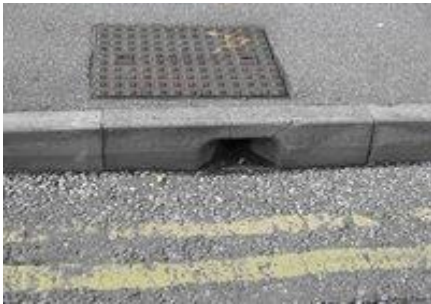
Typical Side Entry Gullies
